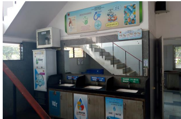
WASH Pledge Model Area – Drinking Water and Hand Wash Station
