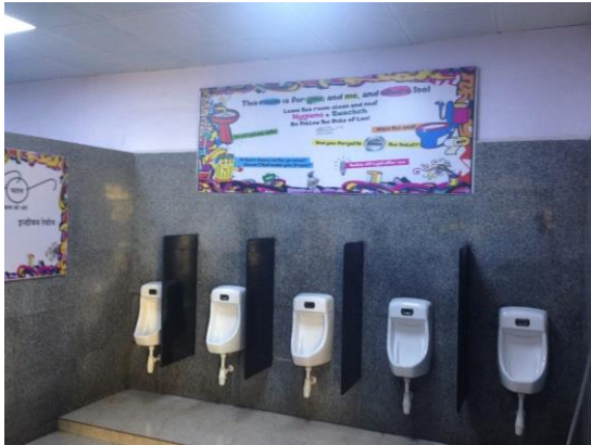
New Urinals Installed with Water Saving Technology
